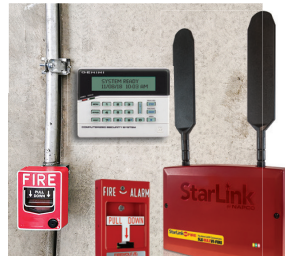
SECURITY & FIRE ALARMS & REPORTING
