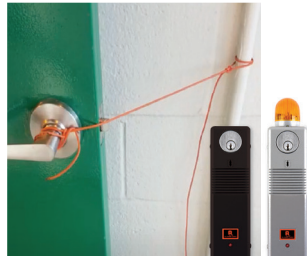
DOOR-PROPPING ALARMS & MONITORING
